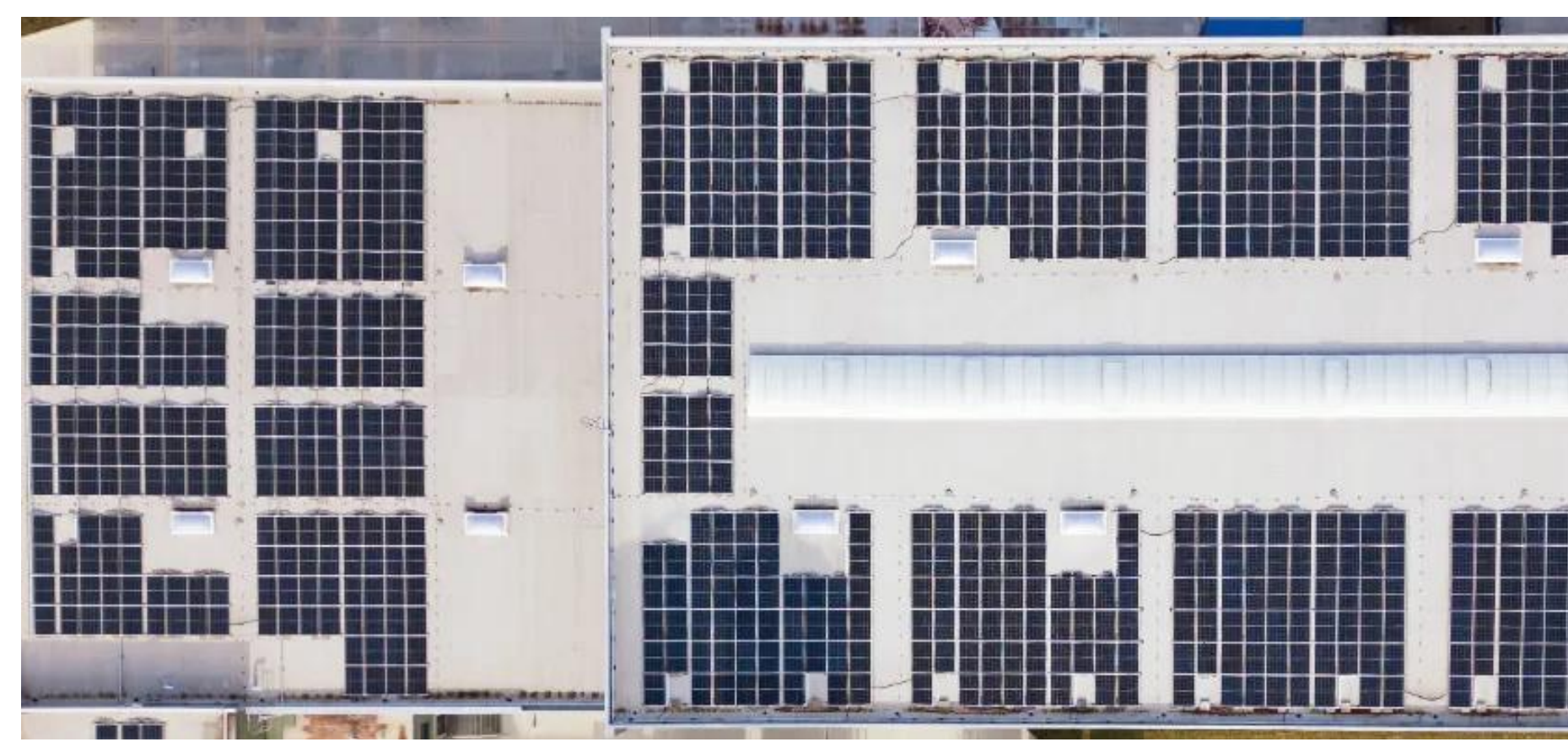
SMS TORK / 610 KWp / 500 kWe / KOCAELİ / 2024
