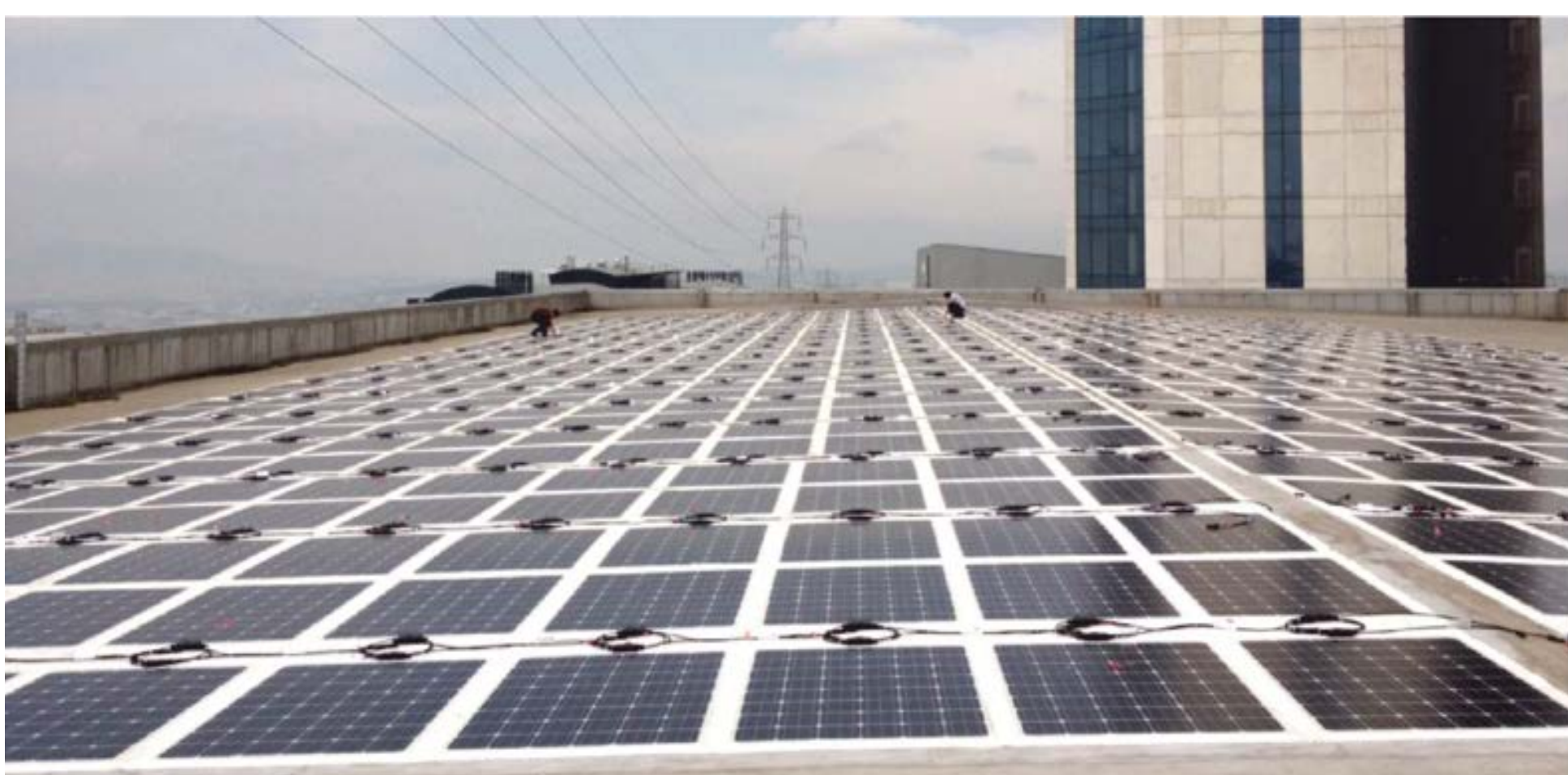
NUH PANEL / 200 KWp / GEBZE / 2016
