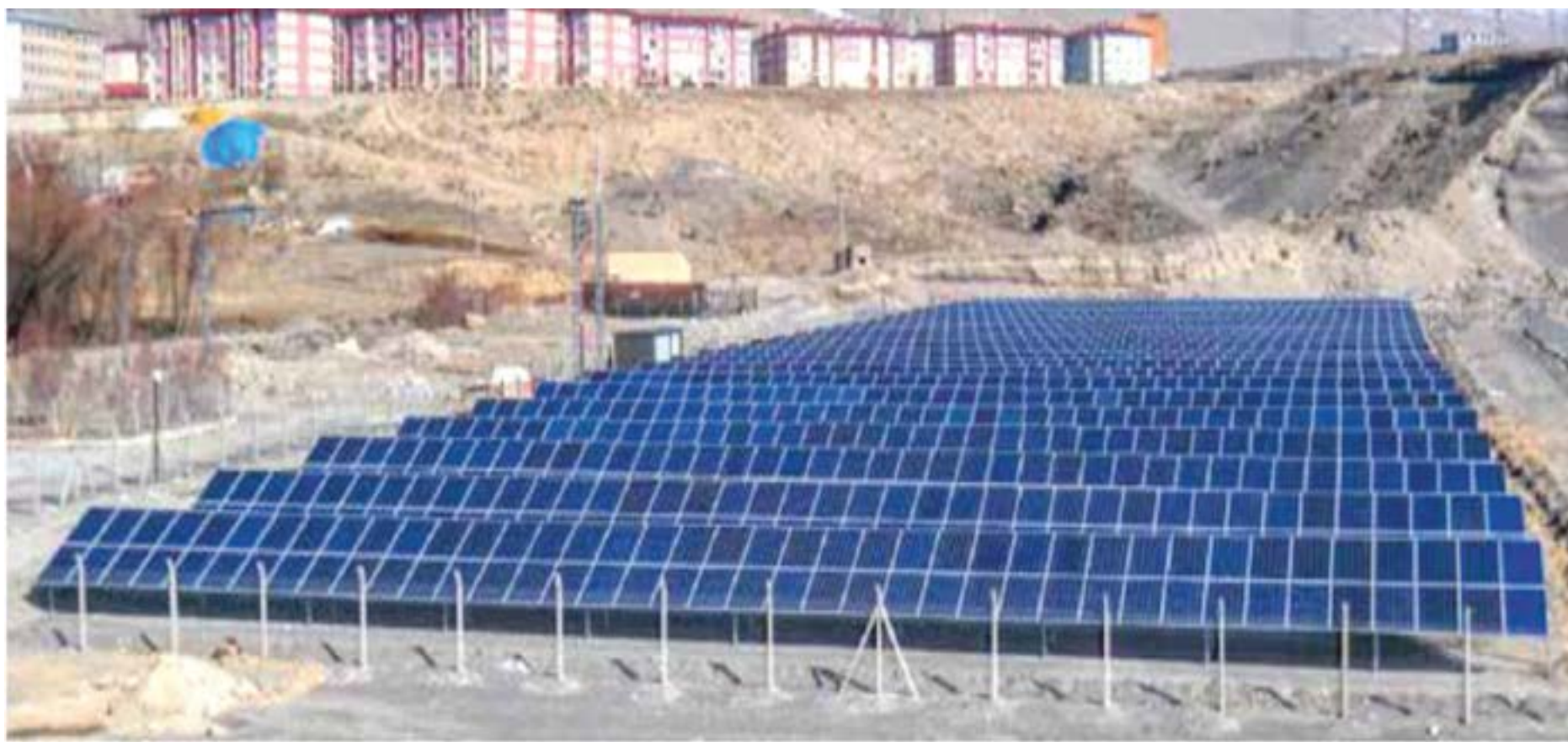
ADİLCEVAZ BLD. / 500 KWp / BİTLİS / 2013
