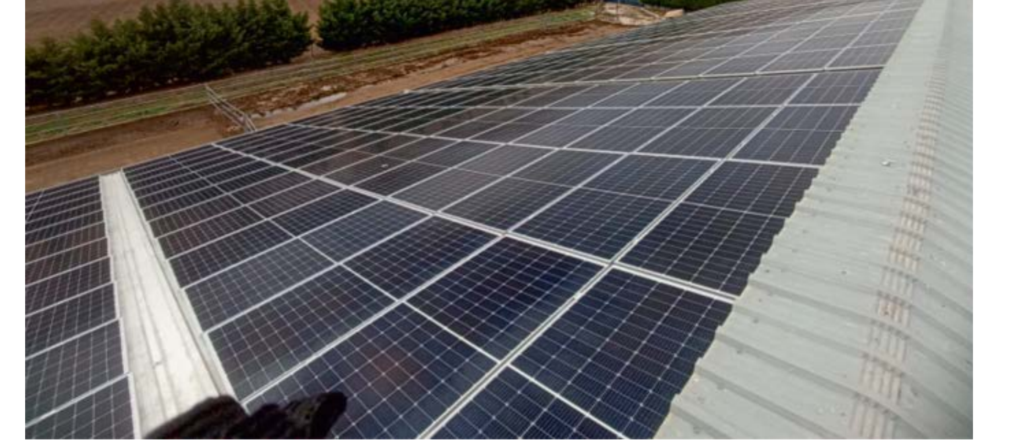
MESA SÜT / 518 KWp / TEKİRDAĞ / 2018
