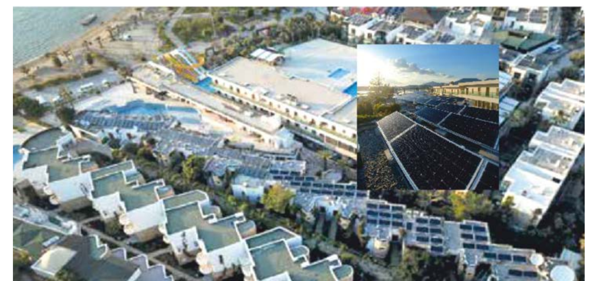
TROPICANA OTEL / 42 KWp / MUĞLA / 2019
