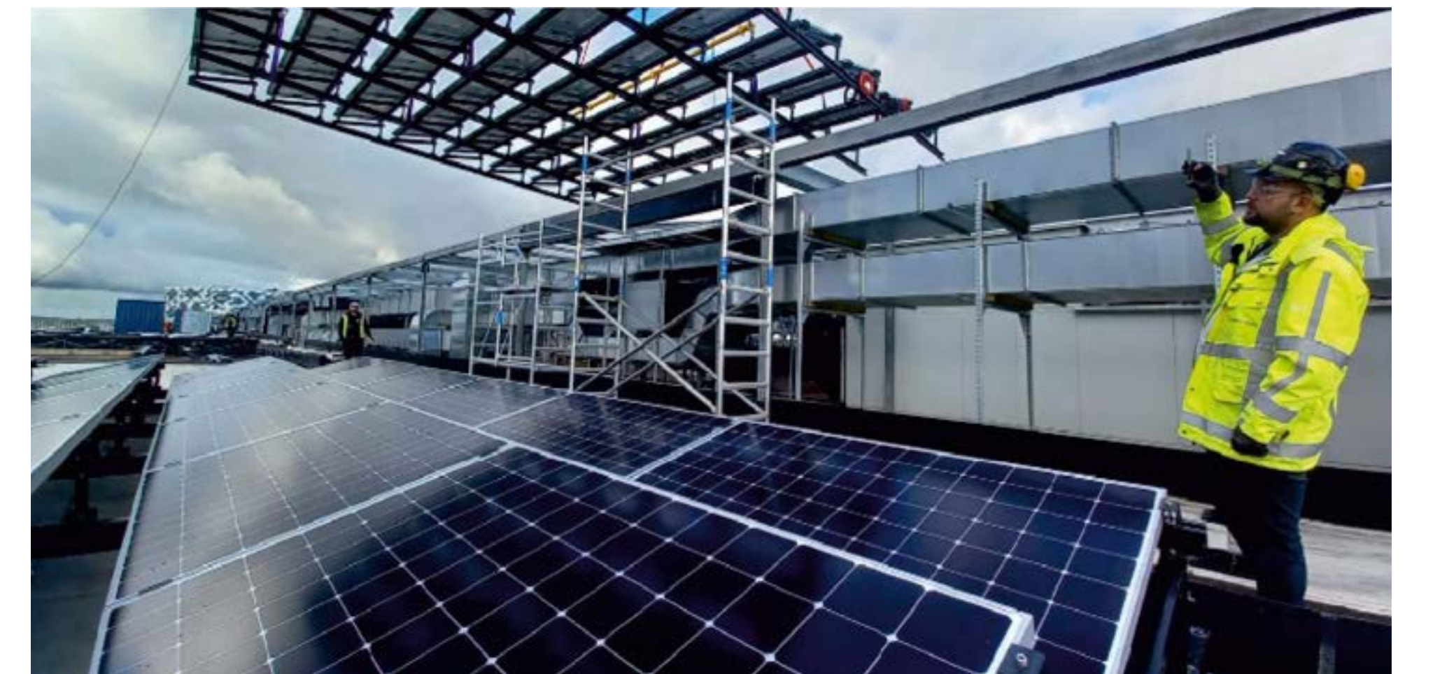
NETHERLANDS SCHIPHOL AIRPORT / 1.2 MWp / NETHERLANDS/ 2020
