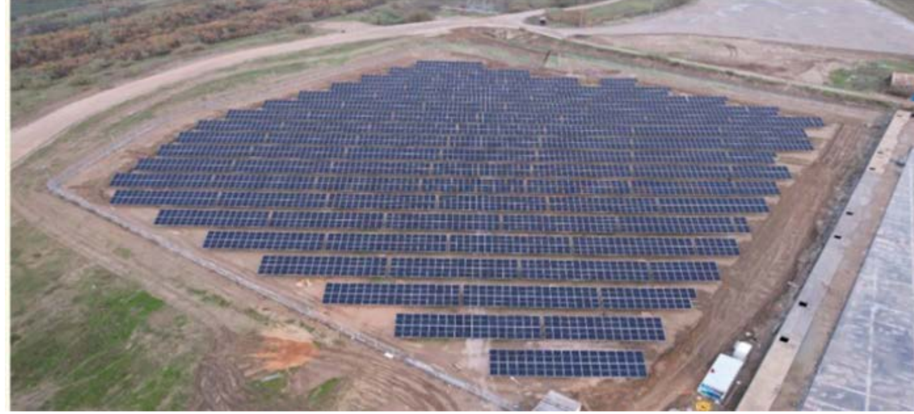
BAĞYURDU OSB GES / 1660 KWp / 1600 KWe / İZMİR / 2023
