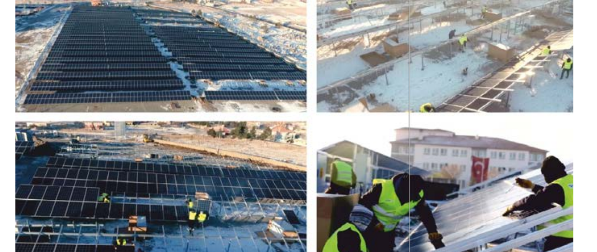
TALAS BELEDİYESİ / 1.15 MWp / KAYSERİ / 2016
