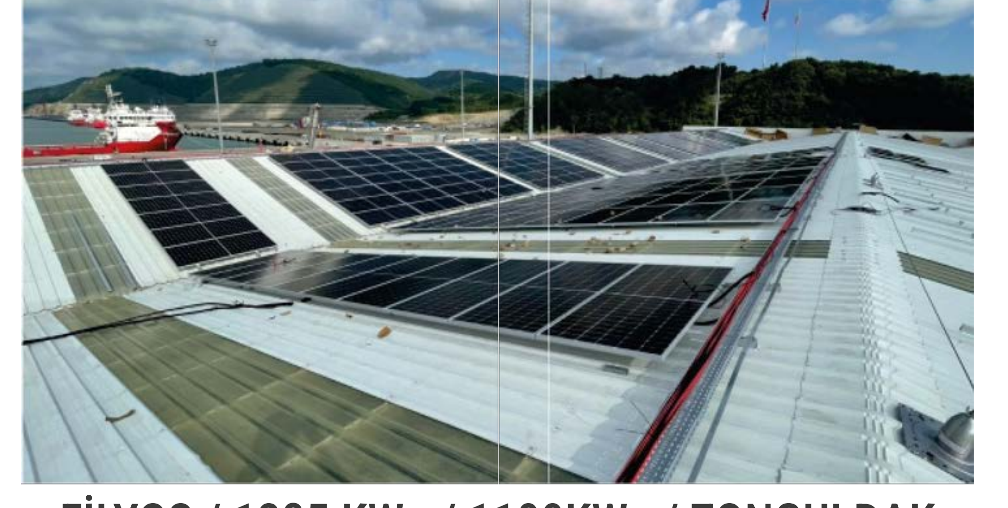
FİLYOS / 1385 KWp / 1100KWe / ZONGULDAK
