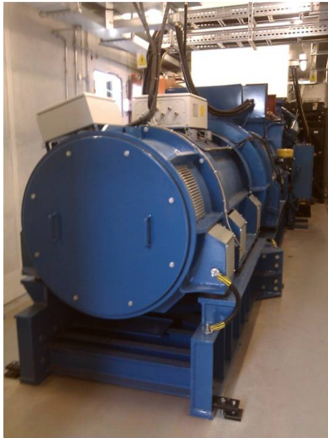
Thames Barrier 2 x 1000kVA
