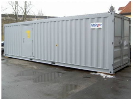
Built into container
