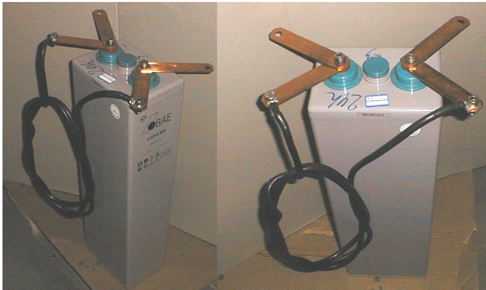
Figure 23 – Bridged 2V 6 OPzV 300 single cell
